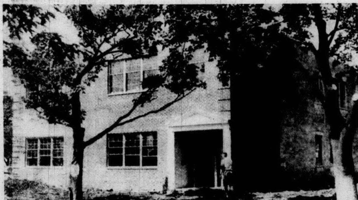
A NEW OFFICE building for the Michigan Bell Telephone company is nearing completion on South Harvey street. The two story building will replace the commercial building on Penniman avenue where phone subscribers transact business. Michigan Bell also has another building on Ann Arbor road in which automatic phone equipment will be installed.
