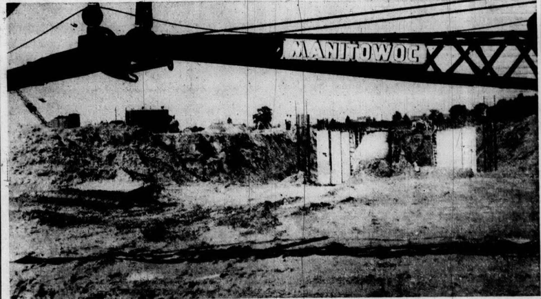
LOOKING UNDER the boom of a large crane, this shot shows some of the activity at the Western Electric Co. plant. Over 600 footers need to be constructed and 87 piers, some of which are shown here. There are 107
