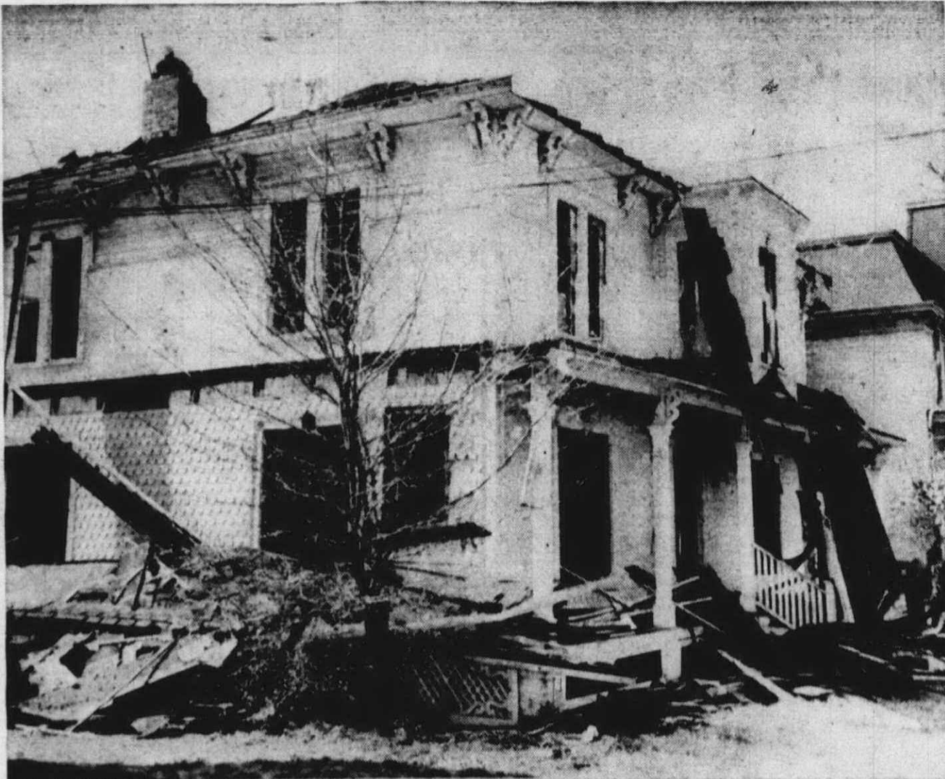
COMING DOWN fast is the old portion of the Plymouth Library which will be replaced with a new colonial structure. A wrecking company moved into the building Wednesday morning and expects to have it almost flattened by Thursday night. The old home has been used as the library since 1945, first on a rental basis and later as a gift from Mrs. Bessie and Miss Margaret Dunning. The new rear addition, completed in 1954, is now housing all library functions. The new unit will be financed by the Edward C. Hough and Mary Hough Kimble Foundation and will cost $116,000.
