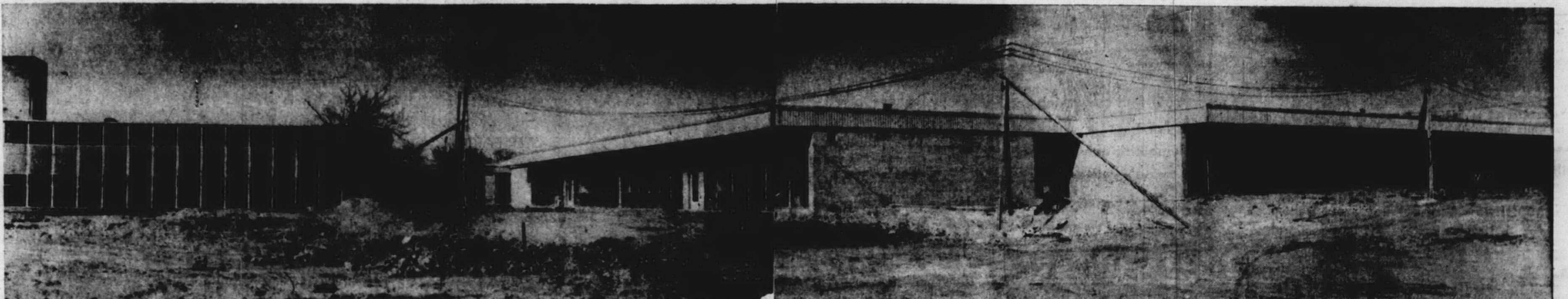
A PANORAMIC VIEW of the Plymouth Community Junior high shows the progress made on the building since ground was broken last year. This view was taken looking north and shows only part of the sprawling building. Being built at a cost of about $1,500,000, it is located west of S. Mill street. It is scheduled to open next fall and will accommodate seventh and eighth grade pupils along with some sixth grades on a temporary basis. The present junior high, located behind the high school, will be renovated for high school use. Money for this work was included in the $3,000,000 bond issue of two years ago. Work on the new junior high continued throughout the winter and is on schedule despite a steel strike.
