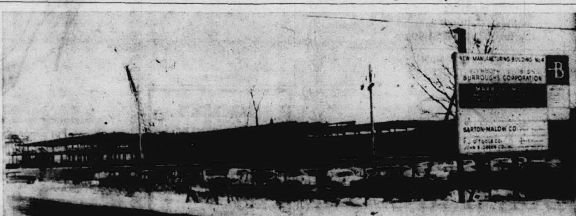
NOW NEARING 50 per cent completion, the new manufacturing building of the Burroughs corporation on Plymouth road is fast taking shape. Steel work is now up and brick laying continues. Scheduled for completion in mid-1957, the new facility will increase the plant's employment by 2,000 by 1958. The 204,000 square foot addition will increase the plant's manufacturing area to 840,000 square feet, or 19 acres. This is the third expansion of the plant since 1950.
