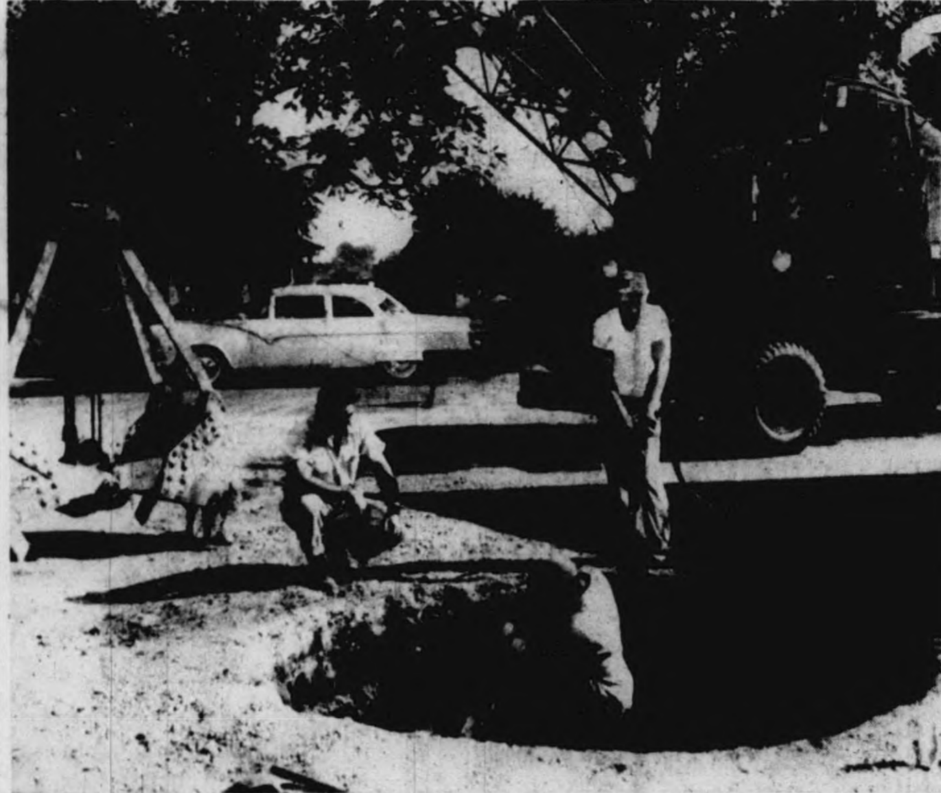
BIRTH OF A $600,000 ditch took place Wednesday morning at Mill street and Ann Arbor Trail. It was the start of the sanitary sewer system that will serve the southern section of the city. It was only last week that the city commission sold the $600,000 bond issue. The contractor, George A. Odien, Inc., started moving the equipment immediately. A manhole 18 feet deep is shown being dug. The new sewer will tap into the old sewer system a few feet beyond this hole.
