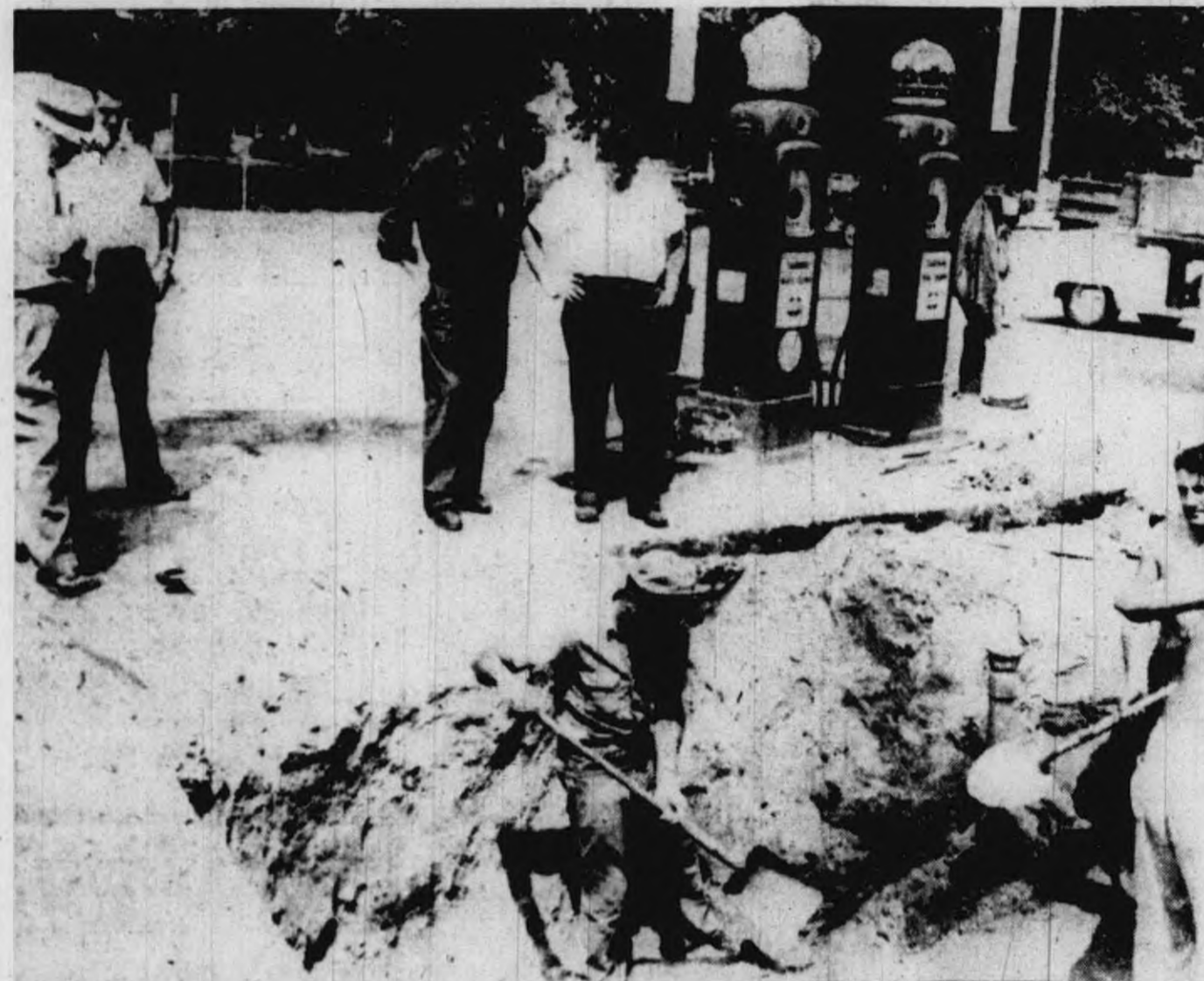
THERE WERE anxious moments Tuesday night and Wednesday when 1,200 gallons of gasoline leaked from an underground tank which workmen are shown digging out. In the center are Fire Chief Robert McAllister and station owner Robert Sincok watching the men dig out the gasoline-soaked sand.
