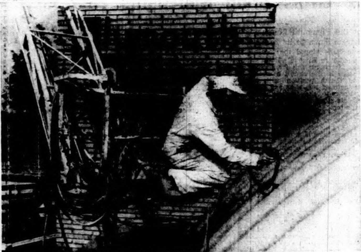
PAINTING FROM his lofty platform is Herb Gilbert, owner of Rainbo Painting Service. With his soaring spray paint rig, Gilbert was giving a coat of vinyl plastic paint to Plymouth Nurseries, 38901 East Ann Arbor road, last week.
