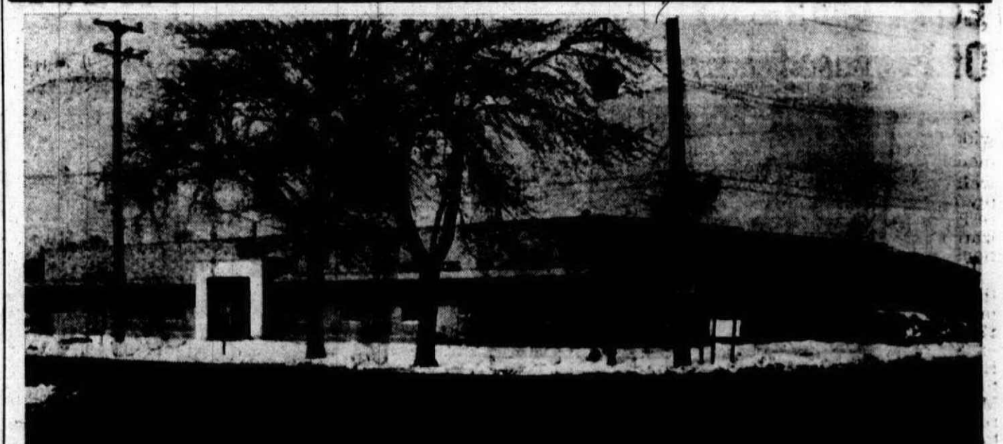
M. POWELL AND SON Stroh's distributor, 110 East Ann Arbor road, is the scene of a major remodeling and building project which will considerably enlarge the original building. A 50' by 100' addition, facing Ann Arbor road, includes these new features: attractive face brick front, marquee, main entrance lobby, offices and a conference room. The project should be completed by spring, according to Mrs. Russell Powell, manager.
