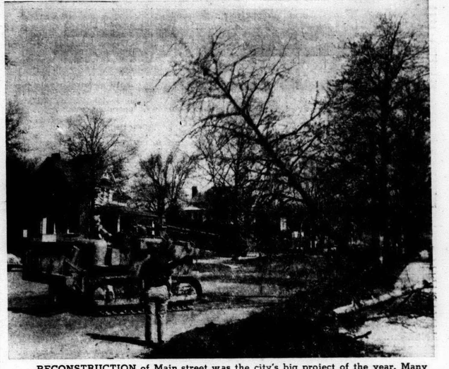
RECONSTRUCTION of Main street was the city's big project of the year. Many trees had to be cut to make way for the widened street. A bulldozer is shown pulling over a tree.
