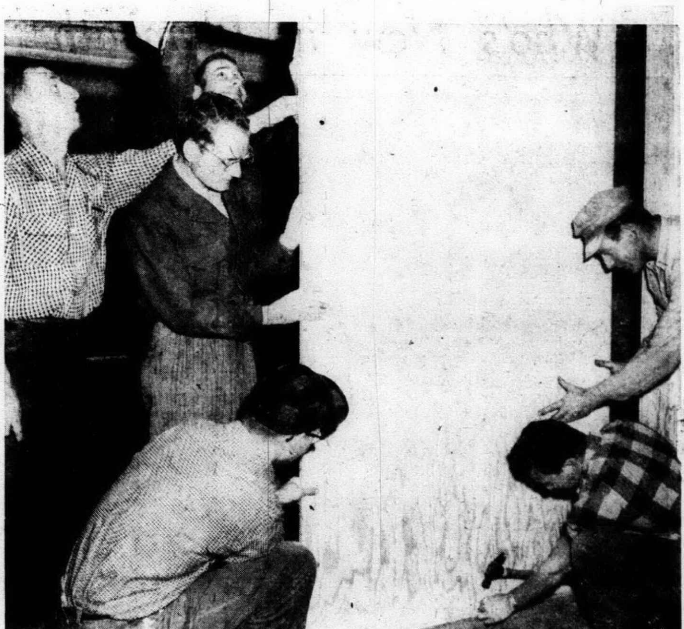
CONSTRUCTION OF nursery rooms was begun last week in Plymouth's newest church, Spring Street Baptist, by members of the local congregation. Partitioning off the basement area above are: Left, reading clockwise, Bill Nipp, Al Moss, Reverend Royall Martin, church pastor; and Percy Owens, Tom Griffin assists Buford Conn at right. An affiliate of the Southern Baptist Ass'n., the church was organized August 28 following a series of tent revival meetings. The growing membership now stands at 67. A choir and visiting program have recently been established. Construction of Sunday School rooms will begin shortly.
