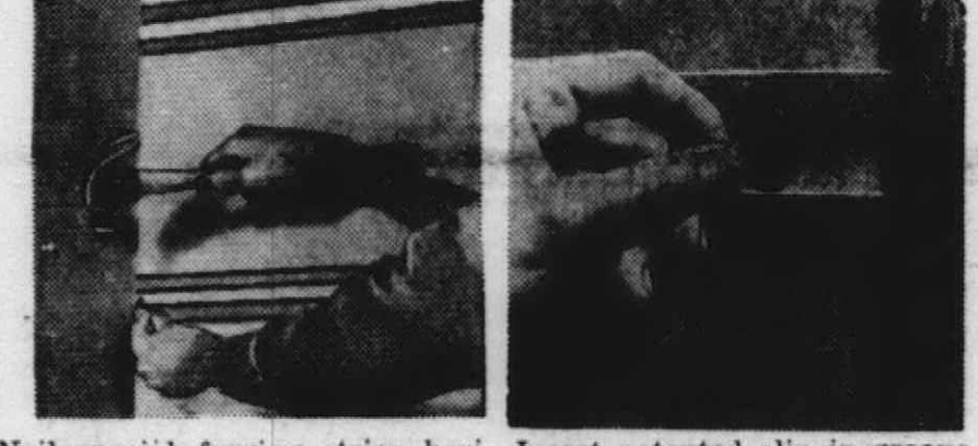
Nail special furring strips horizontally to wall studs. Insert patented clip in groove of each furring strip.
