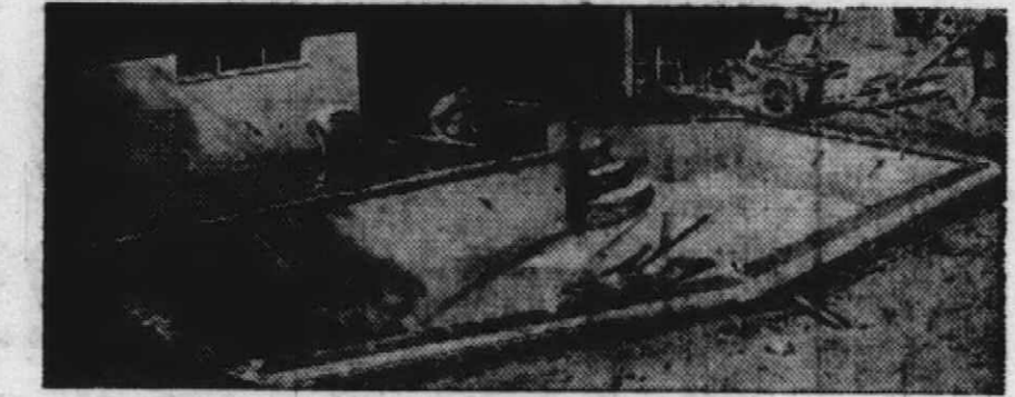
Workmen pour concrete apron as a finishing touch after swimming pool itself has been completed. The pool also is concrete, sprayed on by Gunita process.
