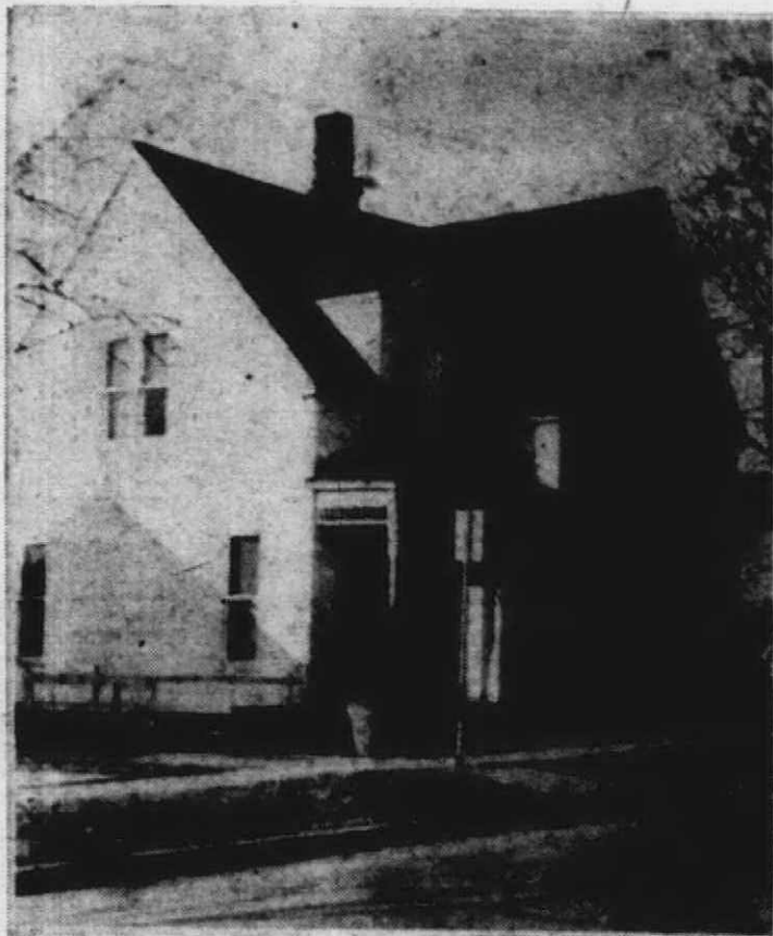
ONLY EIGHT HOURS time were required for a 60 year old Plymouth land mark to be torn down to make way for further commercial development. The Czar Penney home at 498 South Main was totally demolished by a ruthless wrecking crew last Friday. The site next
