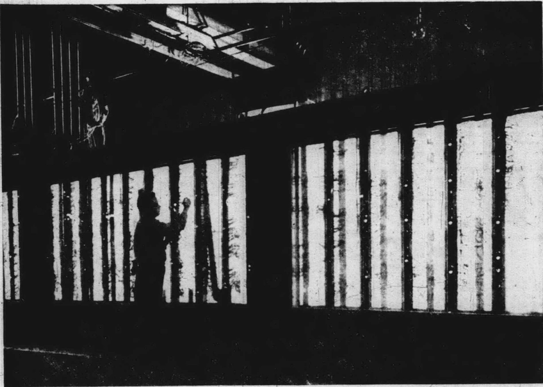
HEART OF THE ELECTRONIC system which controls operation of the world's largest bumper plating facility at Chevrolet's new Livonia Spring and Bumper Plant is a series of upright illuminated panels like the one above. There is a control panel like this for each of the three automatic lines. A total of 710 miles of wiring
