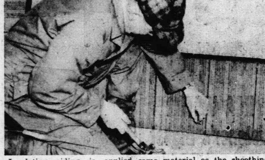
Insulating siding is applied over insulating board sheathing. Plymouth building supply dealers advise using 10 to 14 nails per panel. The siding has a base of insulating board which is the
