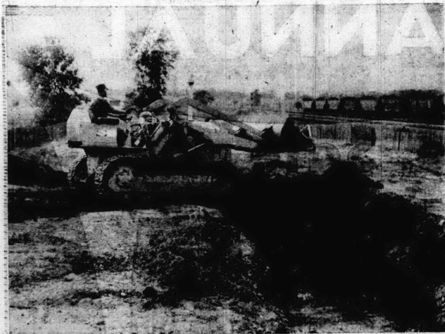
PLYMOUTH NOW USES the "land fill" method of disposing of its garbage, a method becoming widely used after many states, including Michigan, passed laws forbidding the feeding of garbage to hogs. The $11,100 tractor shown here was purchased last month. It digs a trench and buries the garbage soon after it is dumped. Housewives can now follow the previously forbidden practice of wrapping garbage. The land fill site is located at the city garage at the north end of Arthur street.
