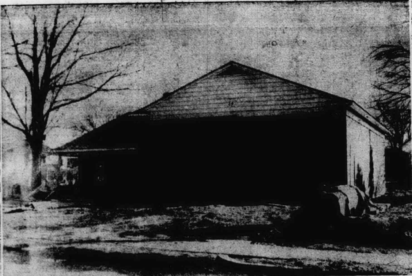
NO, NOT A RANCH STYLE home, but the building shown here is Plymouth's new Northside fire station being constructed at Holbrook and Spring. The colonial structure is now nearing completion and will be occupied within the next few months after the city's new fire truck is delivered. The Burger-Dobbs Construction company of Plymouth started work on the building January 18. Total cost is $18,950.
