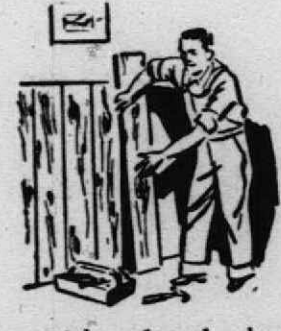
a 2 x 4 must be placed where the wall is slightly concave it may be necessary to place thin strips or "shims" between the 2 x 4 and the wall.
