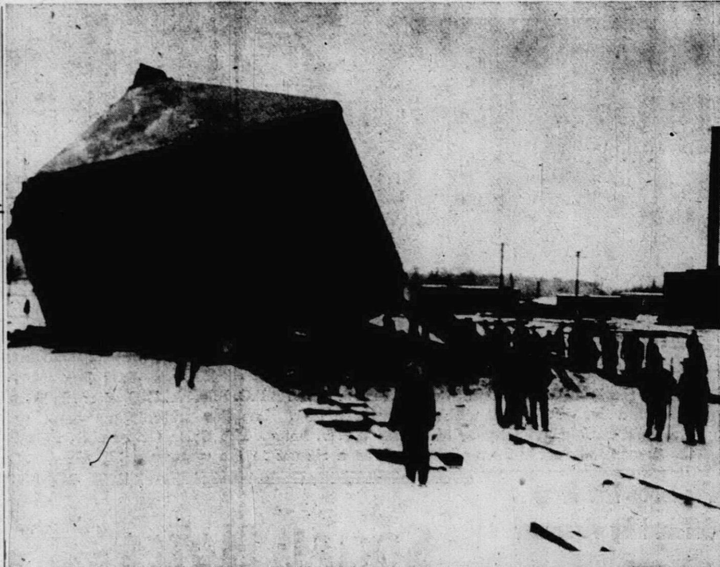
RAILROAD LANDMARK for 32 years, the huge coal hopper in the C & O yards here now lies in ruins after demolition crews finished their work yesterday. The dynamiting of the hopper which took place Tuesday morning was shown on film over a Detroit TV station Tuesday night at 11 o'clock and was pictured in several Detroit newspapers. Top photo taken by The Mail shows the hopper after the blast. Photo at side was taken as the charge went off at 10:25 a.m.
