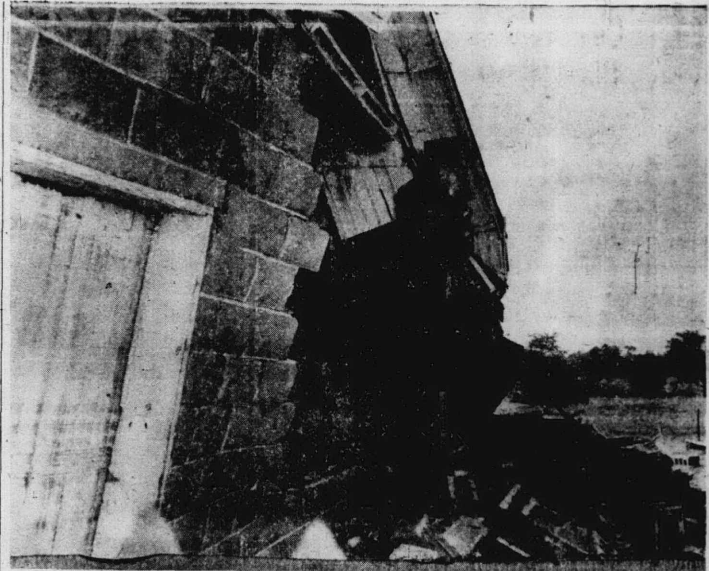
EXPERIENCED FARMERS say that the reason for the collapse of the barn, pictured above, was overloading with hay. The barn, which belongs to Charles H. Bennett, is located on U. S. 12, just west of Plymouth. The hay had been stored there for cattle belonging to Robert Willoughby, who leases the property.
