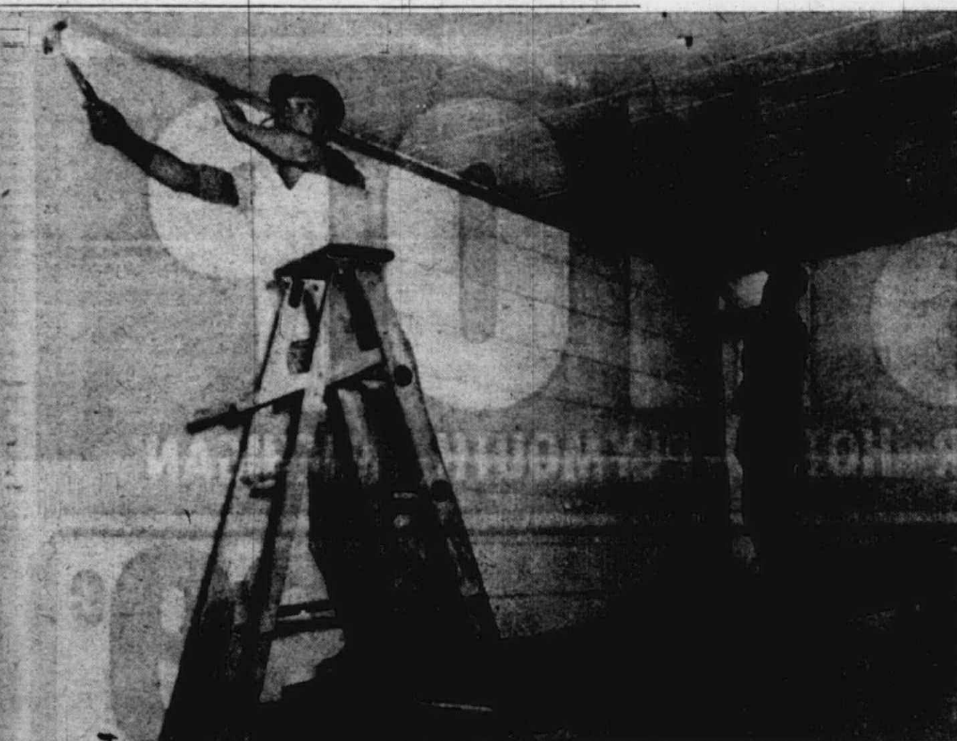
FINISHING TOUCHES are being made on the interior of the Dunning branch of the Wayne County library here by Dick Herrman, left, and Chuck Baumgarten. Details of the construction of the new library are given on page one of this issue.
