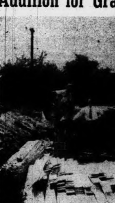
The new Baptist church addition, which Plymouth schools recently leased for classrooms in the fall, is shown above in the process of construction. James Houk, chairman of the church's finance committee, is pictured in the center of the foreground.
