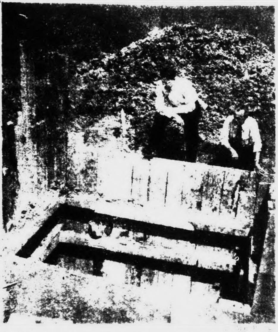
City Manager Harold Cheek, left, and City Engineer Stanford Besse, right, view completion of the first work on Plymouth's new water works improvement plans. It consists of a 50 foot conduit under the railroad tracks on Sheldon road, needed to reinforce the water mains which will later carry Beck road water to the city.
