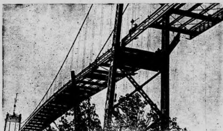
Workmen close the last span in the huge Thousand Island bridge at Alexandria bay, N. Y., which will be dedicated Thursday, August 18 in elaborate ceremonies. President Roosevelt and Prime Minister Mackenzie King of Canada are among notables invited. The bridge crosses the St. Lawrence river and connects Collins Landing, N. Y., with Ivy Lea, Ont. It consists of five spans.
