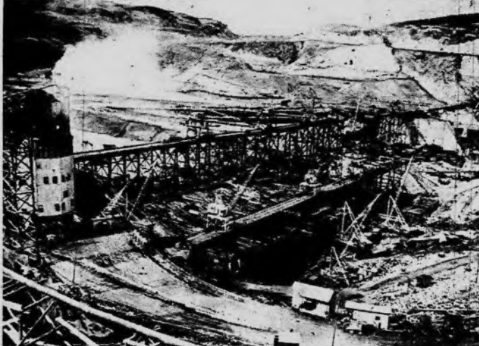
Work is being speeded on the Grand Coulee dam on the Columbia river in the state of Washington, which will eventually cost more than $113,000,000. The giant concrete mixer at left and the second on the opposite side of the river deliver concrete to cars which operate on a trestle. The rising blocks of concrete may be seen below the trestle on both sides.
