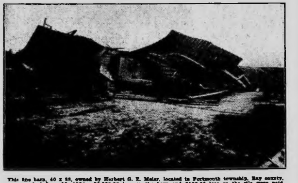
This fine barn, 40 x 88, owned by Herbert G. E. Malar, located in Portsmouth township, Bay county, was wrecked June 10, 1934. $3,800.00 loss on the barn and $100.00 loss on the silo were paid by this Company.
