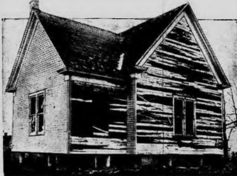
THIS is the Methodist church at Bayville, Mo., after hailstones as large as baseballs and blown by a 60 mile gale had demolished the sides of buildings which were exposed directly to the wind. Weather boarding was smashed, windows broken and shingles torn off.
