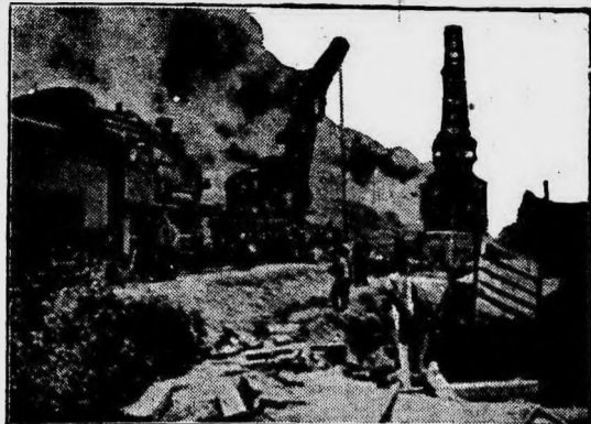
Drawing One of Three Freight Cars Out of a Sink Hole Under the Roadbed of an Eastern Railroad.
