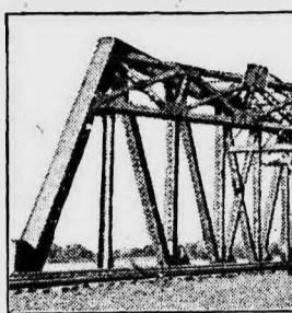
Two Bridges of Different Periods Which Illustrate the Advance Which Has Been Made in Railway Bridge Construction.
