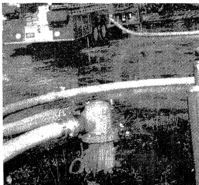
Substantial water pressure finally returned for firefighters around 6 p.m. Sunday night.
