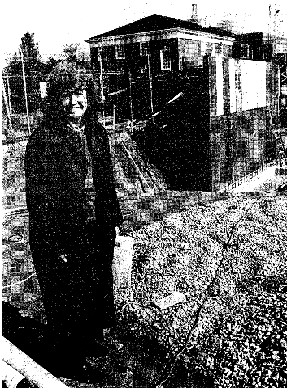
The new Plymouth District Library building is underway. Library Director Patricia Thomas examined the footings and wall forms that are currently being constructed at the Main Street site. The library project is expected to take several years to complete. (Crier photo by R. Alwood Jr.)
