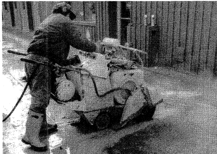
Businesses along Fleet Street in downtown Plymouth got a surprise Monday when utility crews began digging a ditch down the middle of the street. Although the shops face Ann Arbor Trail, most deliveries come through their Fleet Street entrances. (Crier photo by R. Alwood Jr.)
