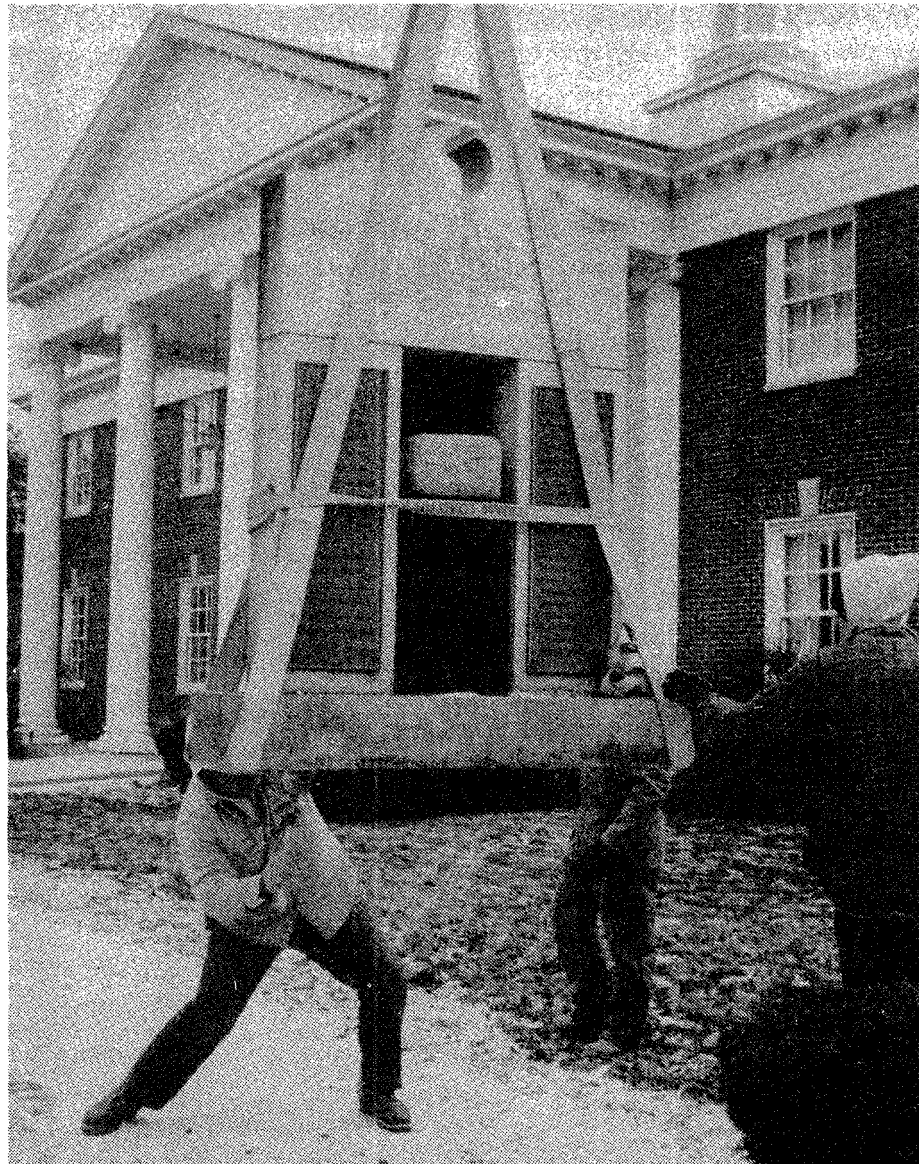
Work crews moved the two-ton Plymouth Rock monument away from what's left of the Plymouth Library. Demolition crews began work clearing the old Dunning-Hough Library to make way for the new structure. (Crier photo by R. Alwood Jr.)
