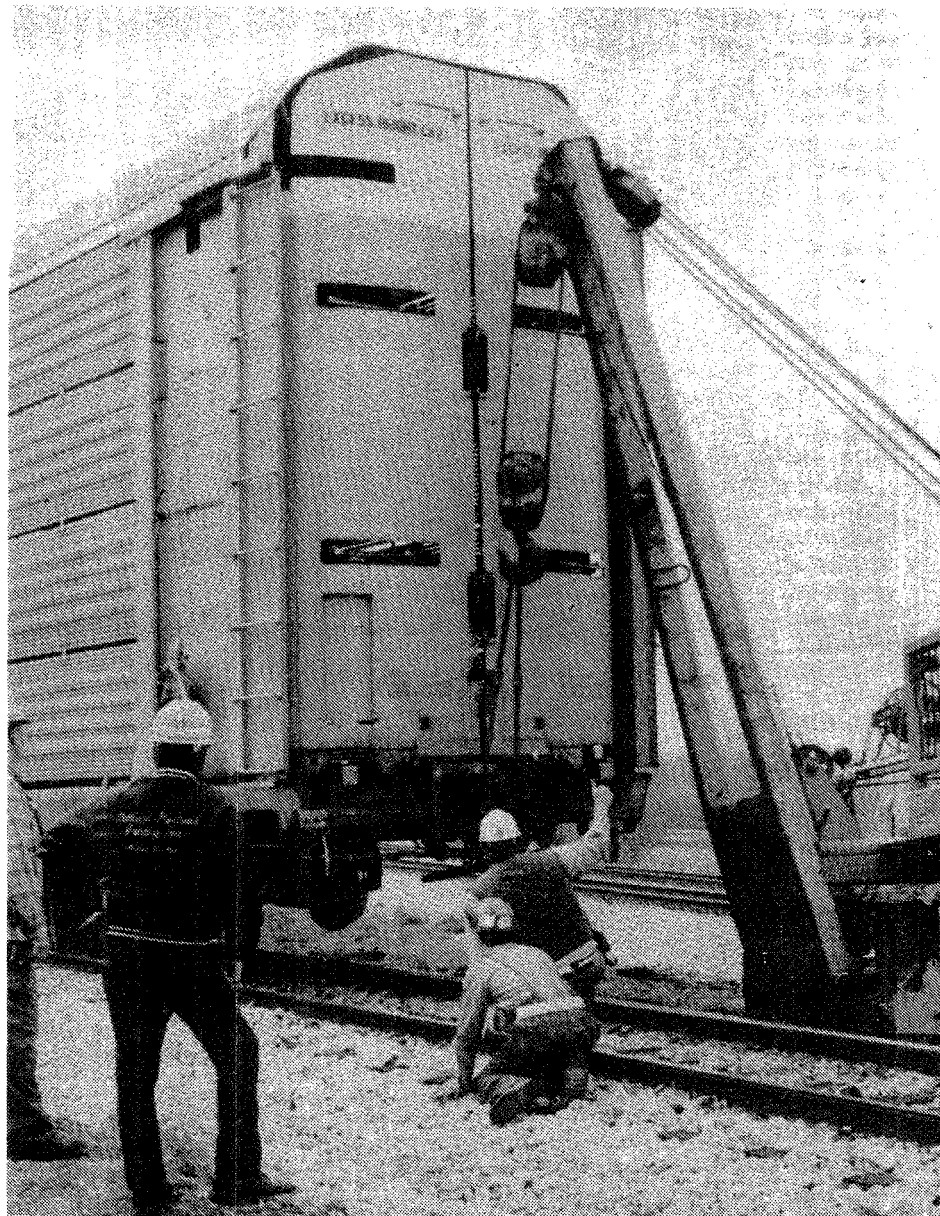
CSX crews worked for nearly 12 hours to get the four cars that derailed back on the train tracks and repair the damaged rail. The derailment occurred next to Station 885. (Crier photo by Stephanie Everitt-Kirkbride)
