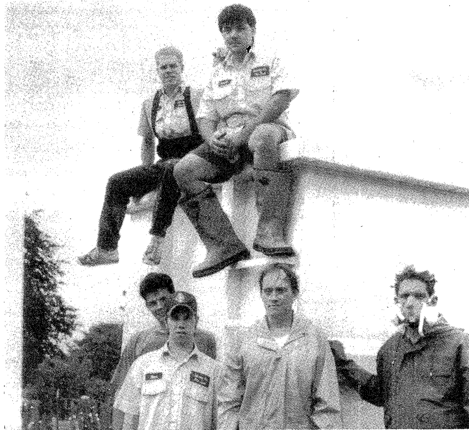
The work crew from Johnny-on-the-Spot takes a well-deserved break after removing raw sewage from the basement of Saxton's Garden Center. (Crier photo by Rob Kirkbride)
