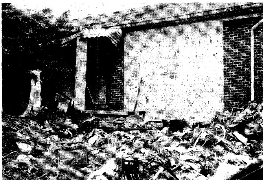
Debris fills the front yard of this house on Michigan Avenue. Although no one was home, the house was filled with items belonging to an elderly woman who was in the process of moving out. (Crier photo by Alex Lundberg)
